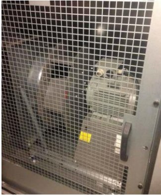
Pump of the ventilation system has to stay clean.
